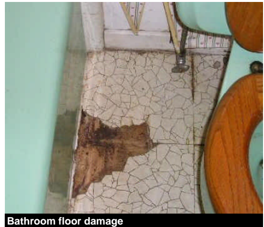
Bathroom floor damage
